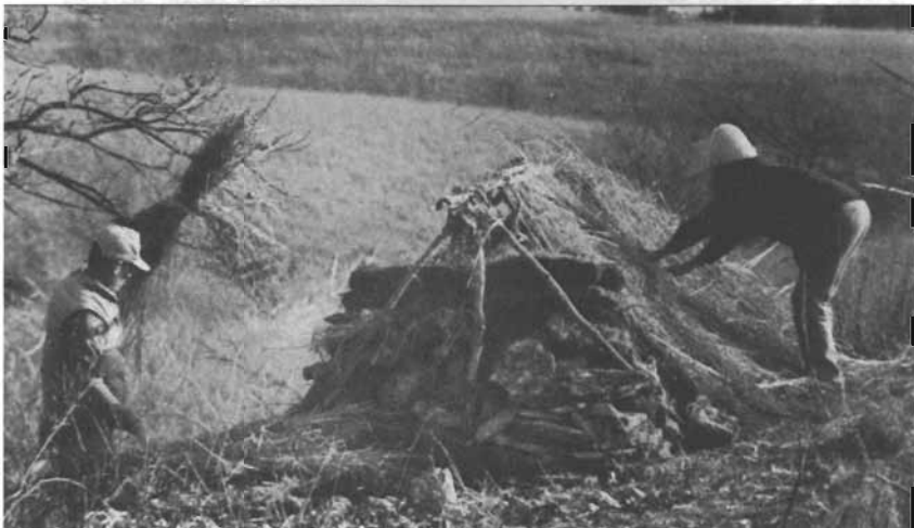
Long grasses are placed on the roof, overlapping the sides and several inches thick. Some pieces of bark are placed on the very peak to help this vulnerable area to shed water.
